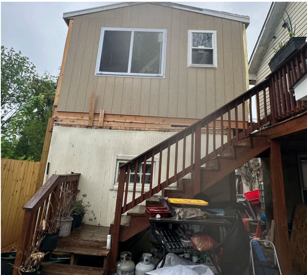
Photo of the constructed shed addition on the Property (provided by Applicant)
