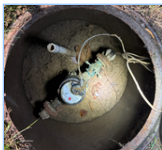
Residential water meter within meter pit
