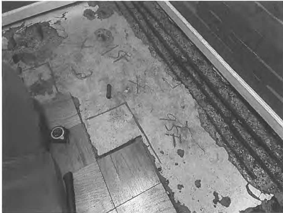
Photo 2 – View of Spalled Concrete and Exposed Corroded Embedded Reinforcing
