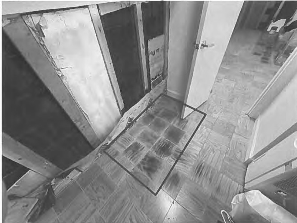
Photo 6 – View of Discoloring of the Wood Flooring in the Walk-In-Closet
