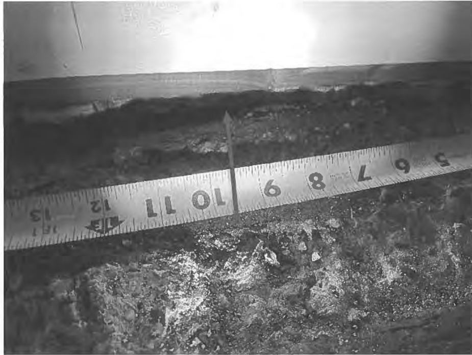
Photo 6 – Leak Noted at the Base of the North WIC Wall
