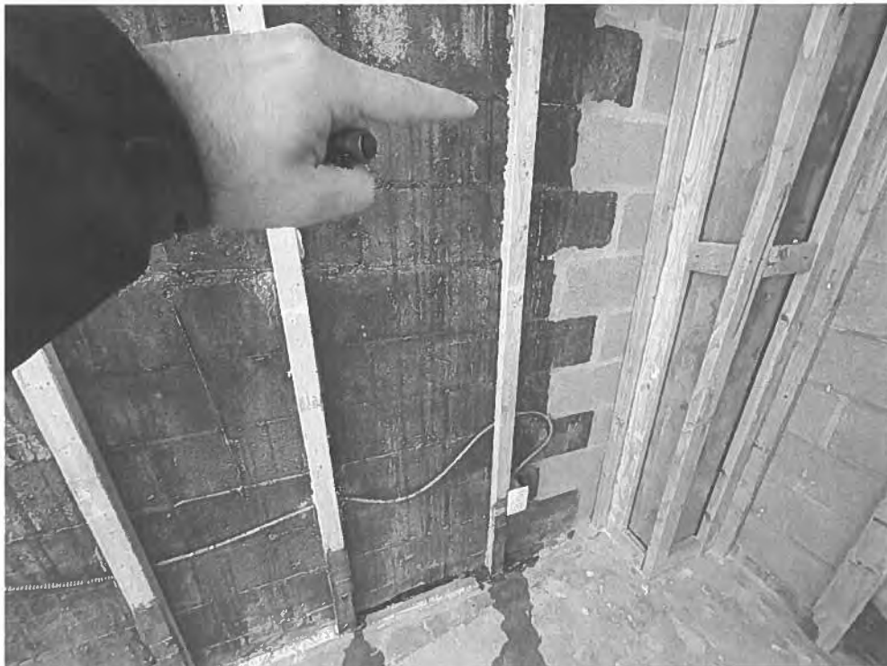
Photo 3 – Water Infiltration Noted at Several Isolated Locations in the North Back-Up Wall
