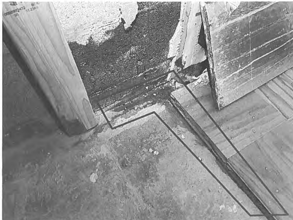
Photo 1 – View of Water Infiltration Observed in the East Wall Due to Past Rain Event
