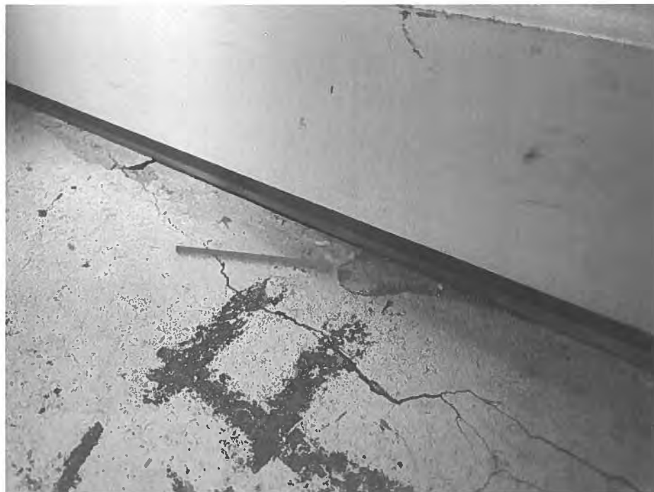
Photo 5 – Leak Noted in the WIC at the Base of the West Wall
