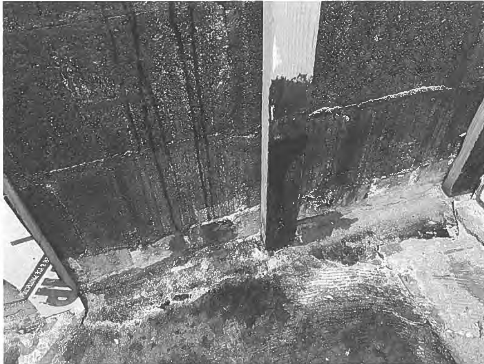
Photo 8 – View of Water Infiltration into the Walk-In-Closet Space
