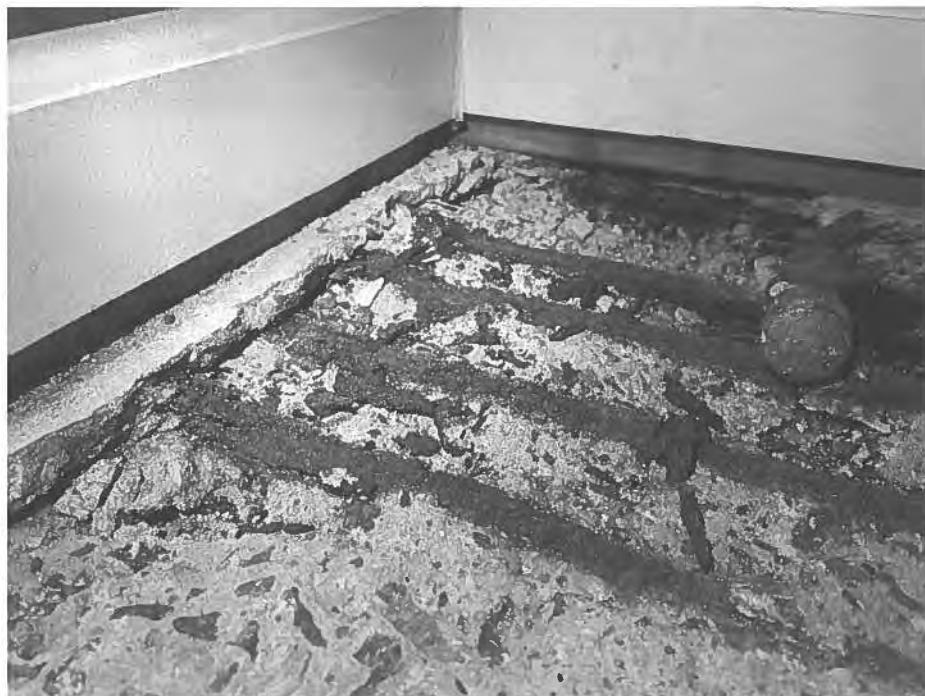
Photo 3 – Close-Up View of Severely Corroded Reinforcement
