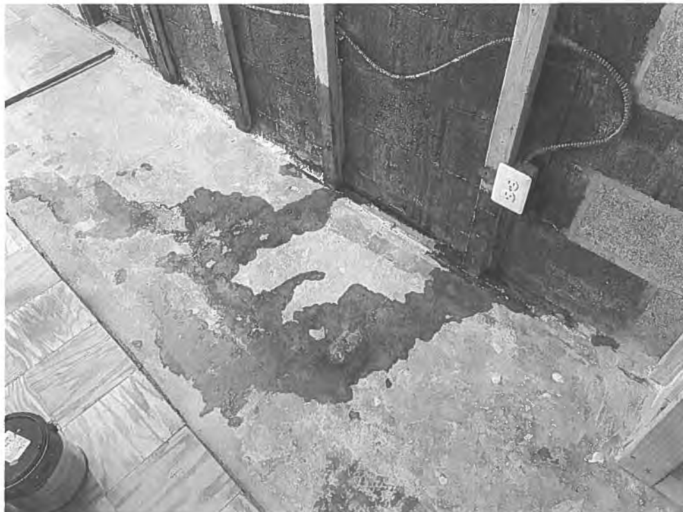
Photo 5 – View of Water Infiltration in the Occupied Space at the End of the Water Test
