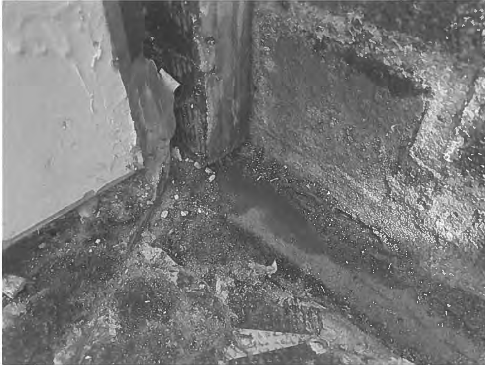
Photo 9 – View of Water Infiltration into the Walk-In-Closet Space
