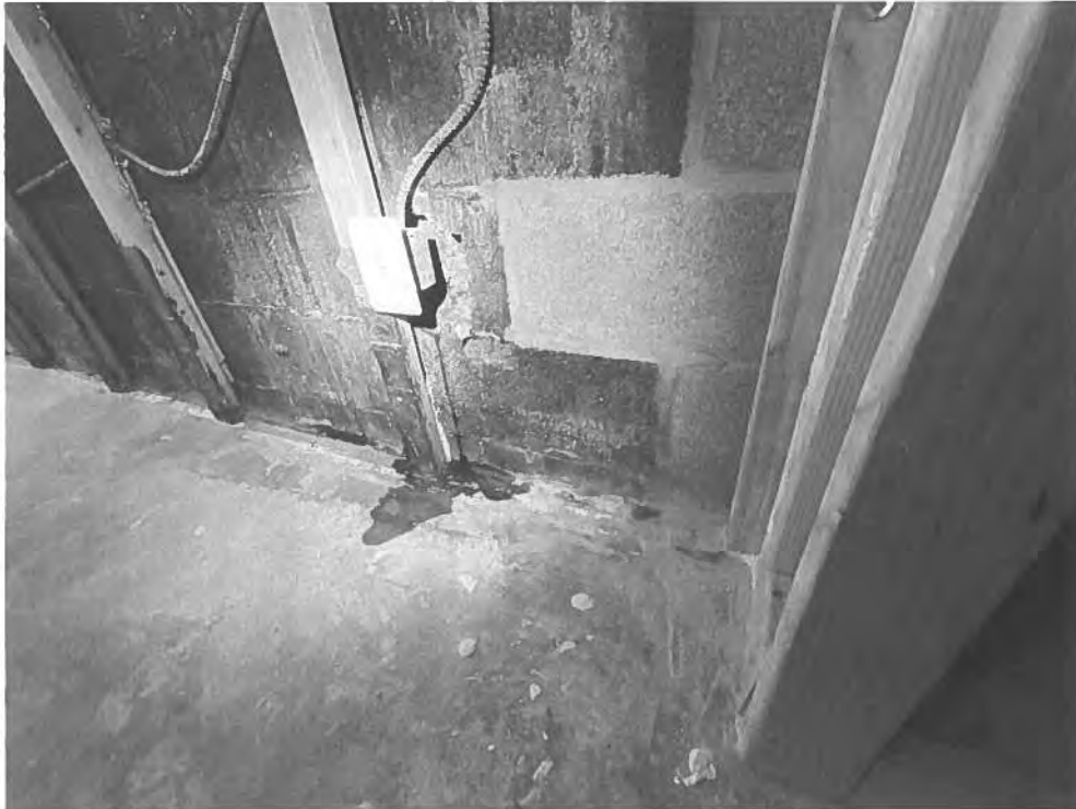
Photo 2 – View of Water Infiltration During Testing of Section #3 on the North Wall
