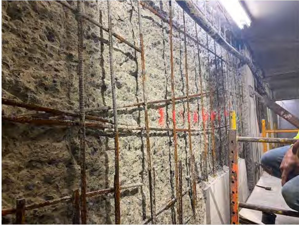
Photo 4: Typical Existing Rebars Marked in Orange for Replacement Due to Significant Section Loss
