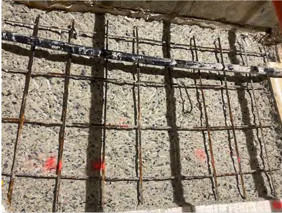
Photo 3: Typical Existing Rebars Marked in Orange for Replacement Due to Significant Section Loss
