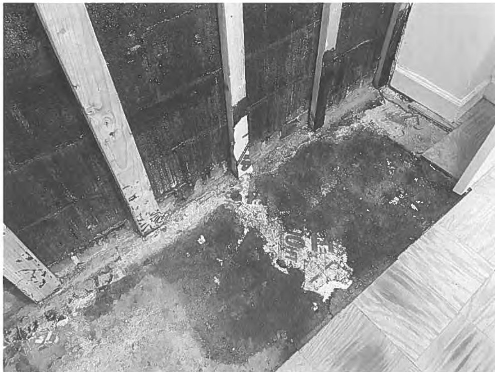
Photo 7 – View of Vegetative Growth Under the Wood Flooring
