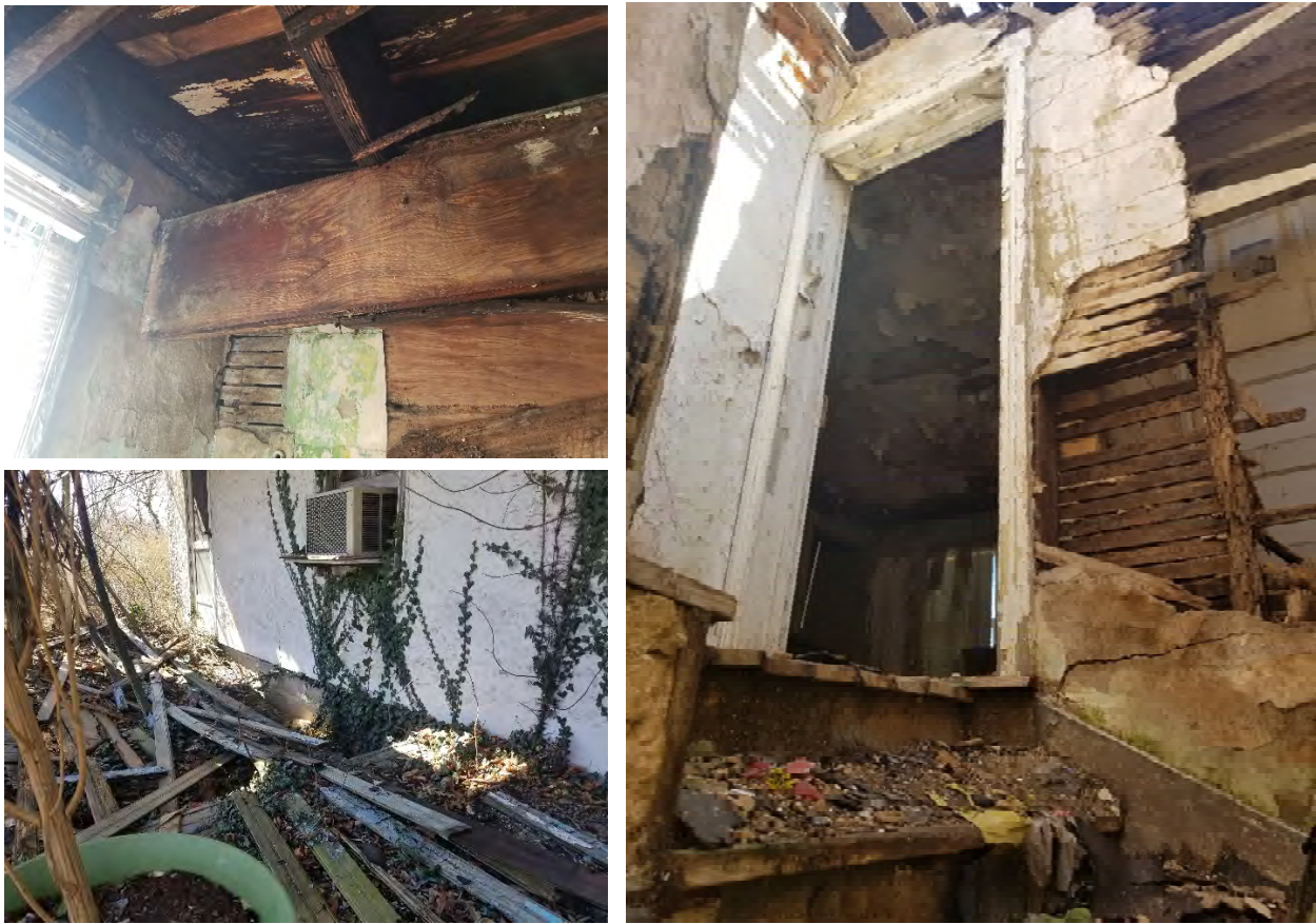
Figure 3 – Extensive damage to the structure
